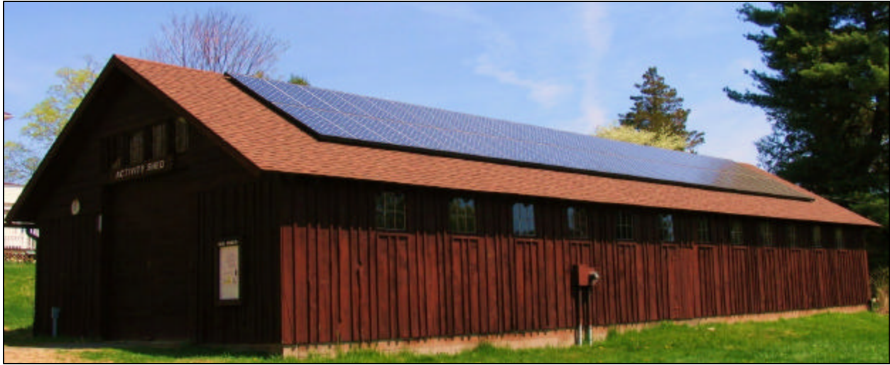
We've Got the Power!: Solar Panels on Our Activity Shed, Photo Credit: Gerri Griswold
